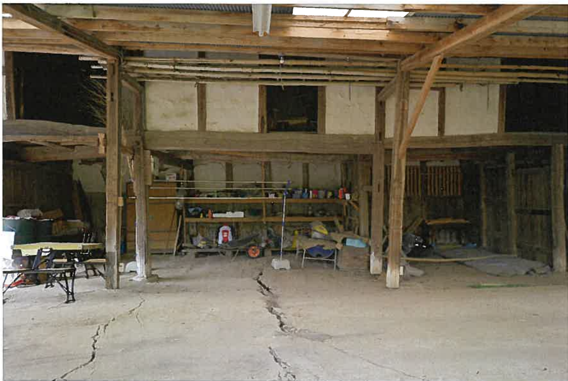
The crack in the barn of a Yano Residence, Nishihara Village, Kumamoto Prefecture
